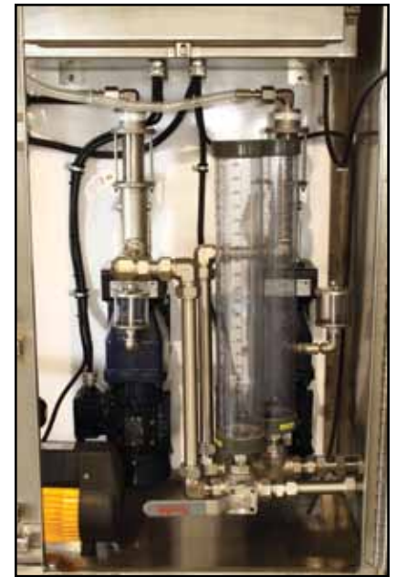
Figure 15 – Select Flocc Dual Polymer PC Feed Pumps
