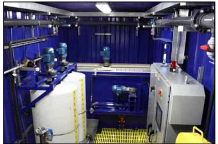
Figure 9a and 9b – KEMTRON DFD Polymer Injection and Conditioning Manifolds
