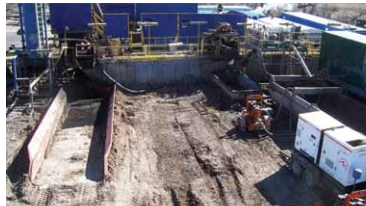
Figure 5 – KEMTRON's DFD System Using a Dry Reserve Pit.
