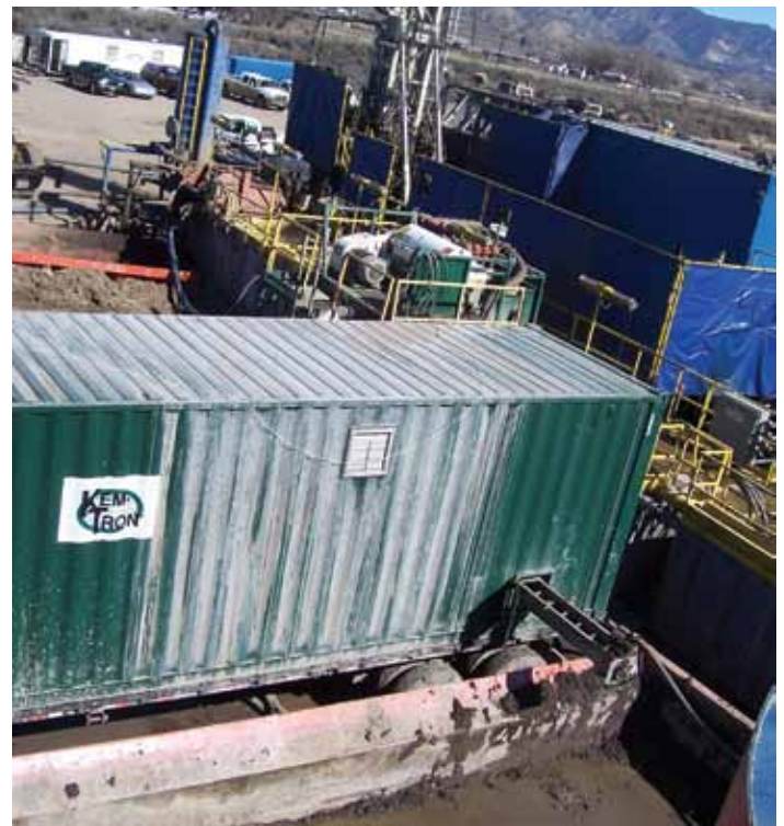
Figure 1 – Land-Based Drilling Fluid Management System Using KEMTRON's KT-DW-40 Trailer-Mounted Dewatering System & KT-1448 Solids Control Centrifuges
