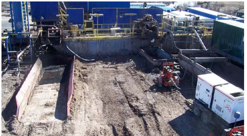
Figure 5 – KEM-TRON’s DFD System Using a Dry Reserve Pit.
