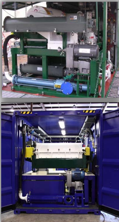
Figure 8 – 20' DFD Systems Fed Via Progressive Cavity Pumps
