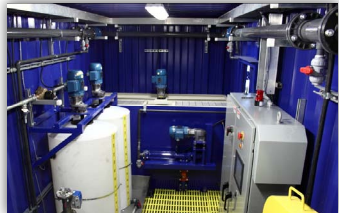
Figure 9a and 9b – KEM-TRON DFD Polymer Injection and Conditioning Manifolds
