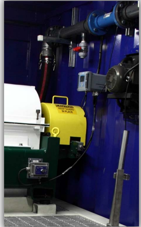
Figure 15– KEM-TRON's DFD Systems Incorporating a HACH Turbidity Meter
